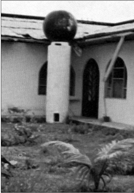
The courtyard of the hotel Victoria Regia. The tower-like structure was supposed to store water but it was usually bone-dry.
